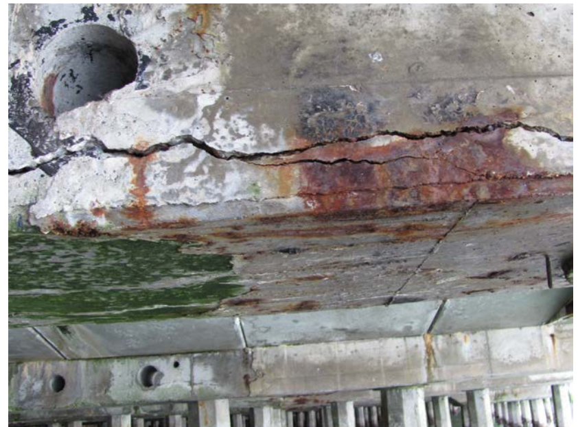
Sample Deck Panel Damages
