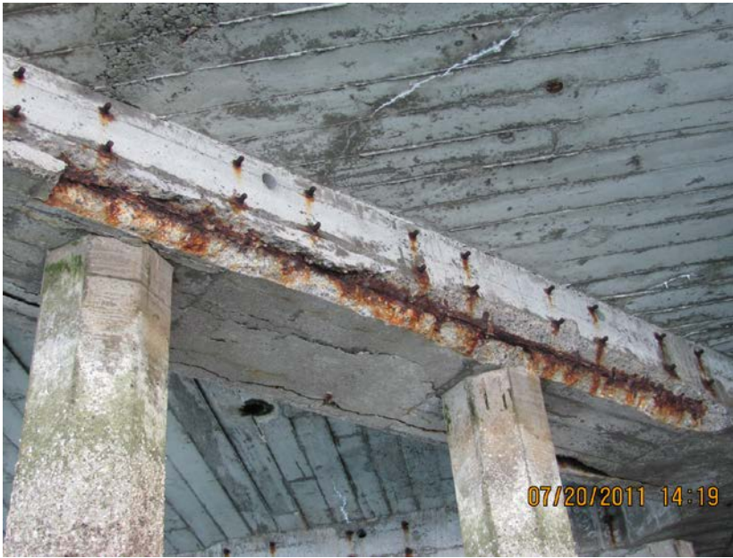
Sample Pile Cap Damages
